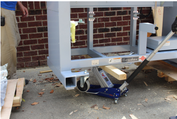
14. Using a good quality floor jack, carefully raise up one end of the machine just enough to remove the pallet. Attach the wheels.
