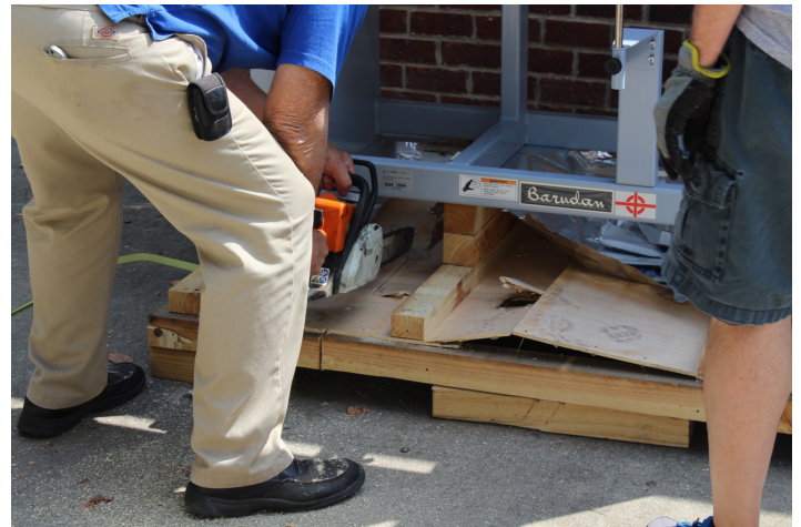
11. If you do not have access to a forklift, carefully cut out the center of the pallet with a chain saw or reciprocating saw.
